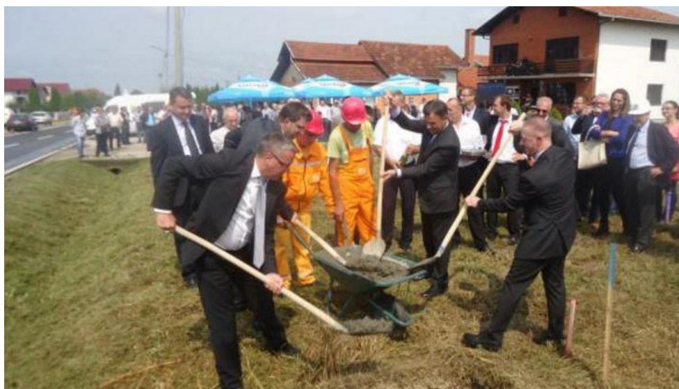
Laying the foundation stone of the Brcko bypass (September 2015). Works are ongoing. The EU has contributed a €0.5 million project implementation support grant.
